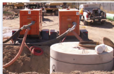
Bypass pumps & manhole
